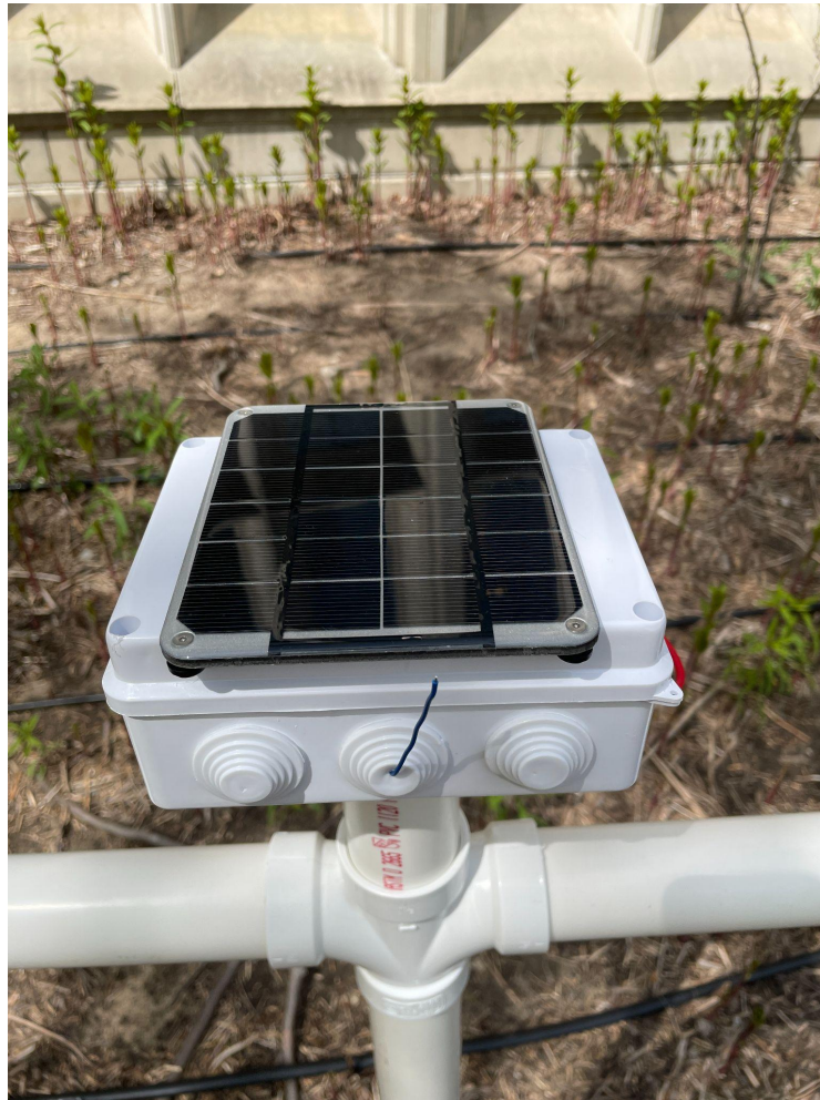
Figure 7. Solar Panel on the Enclosure
